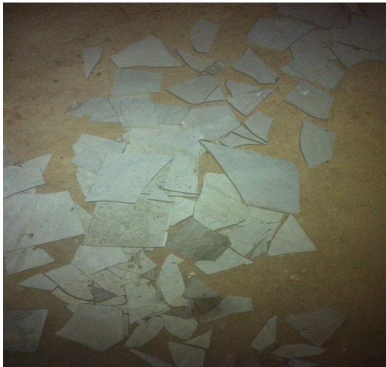
Figure.3. 1.broken tiles available on site
